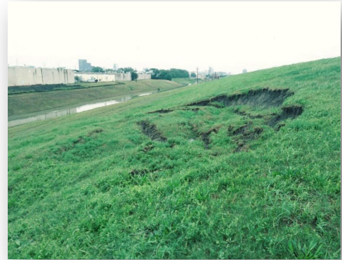
FIGURE 7-7: SLOPE FAILURE OF LEVEE
