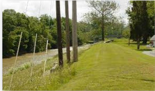
FIGURE 7-9: UTILITY POLES INSTALLED WITHIN LEVEE EASEMENT(UNACCEPTABLE)
