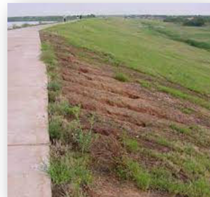
FIGURE 7-8: EROSION ON LEVEE DUE TO RAIN RUN-OFF
